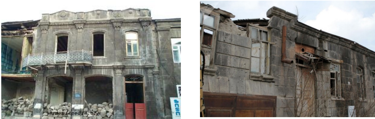
Fig. 2. Destroyed condition of buildings in “Kumayri”
